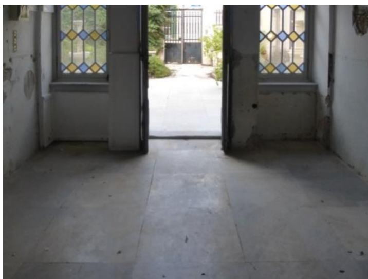
Fig. 4: Marble floor slabs 74x74 cm at the entrance, lined up to the relevant at the yard. Source: G. Antoniou, 2015
